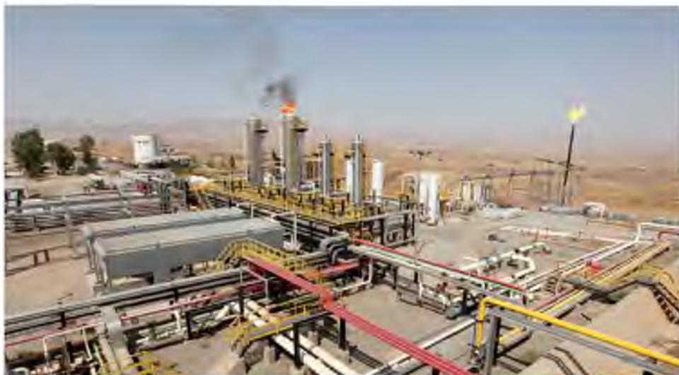
A flame rises from a chimney at Taq Taq oil field in Erbil, in Iraq's Kurdistan region, Aug. 16, 2014. REUTERS/Azad Lashkari
