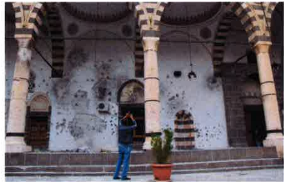
A man takes pictures of the damaged walls of a mosque with his mobile phone in Sur district in the Kurdish dominated southeastern city of Diyarbakir, Turkey, in this October 13, 2015 file photo.
