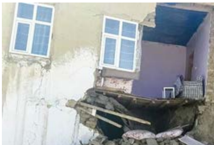
Firefighters respond to damaged buildings after an earthquake struck the eastern city of Van. Photo: Nihat Ozbey / IHA
