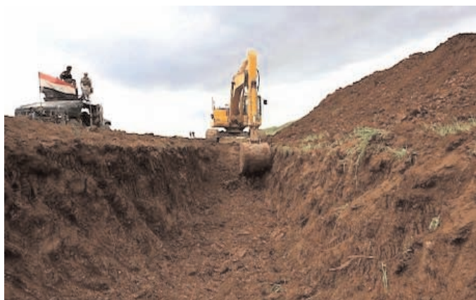
Officials say the trench is three meters wide and two meters deep, aimed at preventing smugglers and terrorists from infiltrating into Kurdistan. Photo: Rudaw
